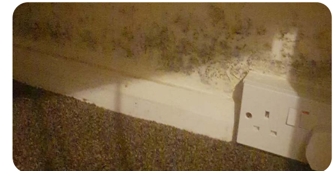
Damp in the home
